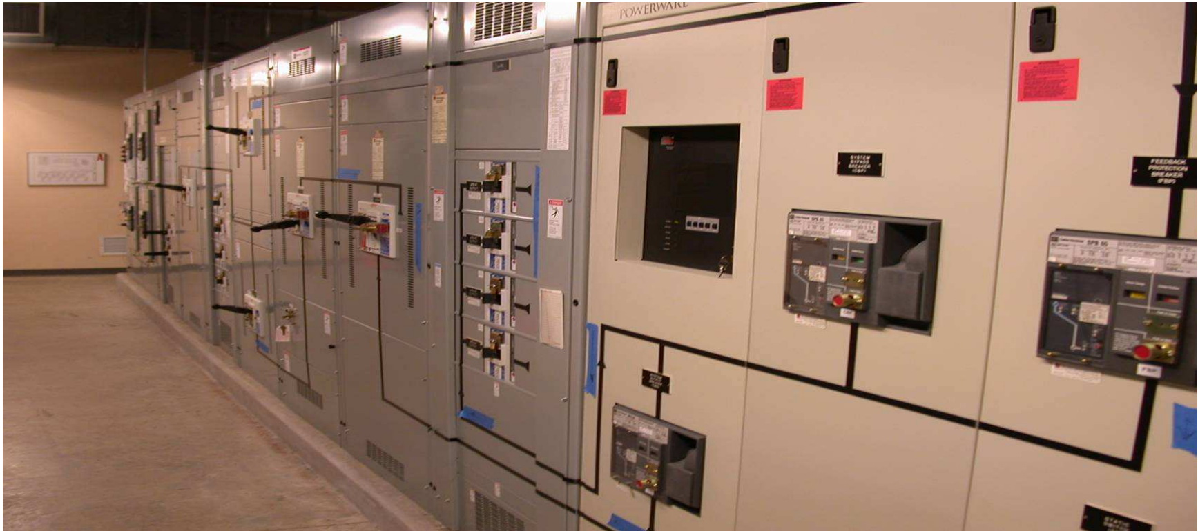
Emergency Power Switch
