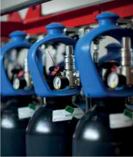
Sophisticated fire suppression system
