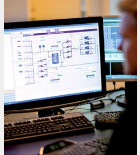
Monitoring from the Network operations Centre
