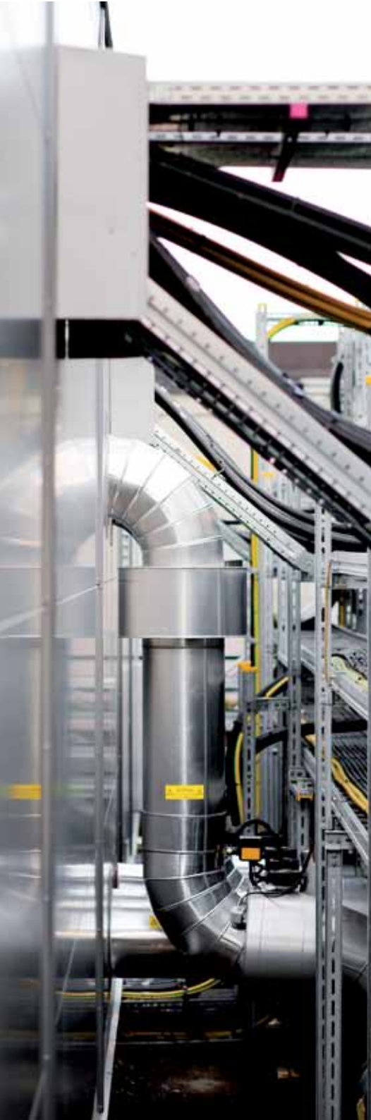
Chilled water pipes
